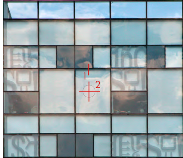
Fig. 2: The curtain wall system seen from the outside on the west side of the building. A temperature sensor was lowered into the air cavity through a 1/4 inch hole at position 1. The tip of the sensor was placed at position 2.
